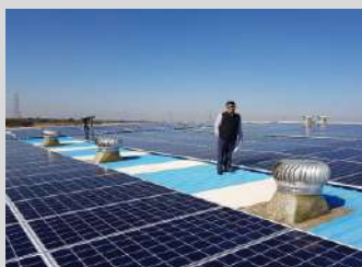
500 kW (Jaipur - Rajasthan)
