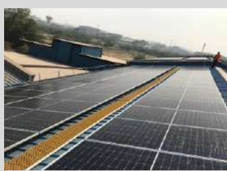
1 MW (Ahmedabad - Gujarat)
