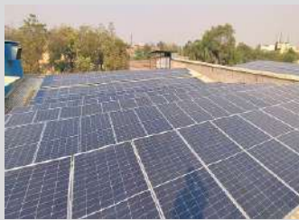
550 kW (Ahmedabad - Gujarat)
