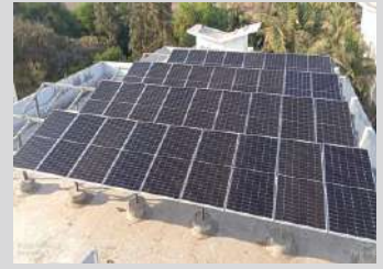
600 kW (Gandhinagar - Gujarat)
