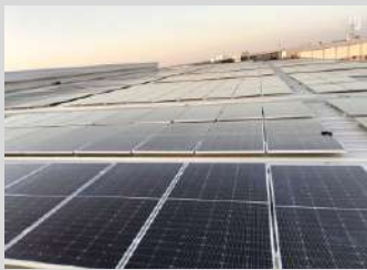
600 kW (Jaipur - Rajasthan)
