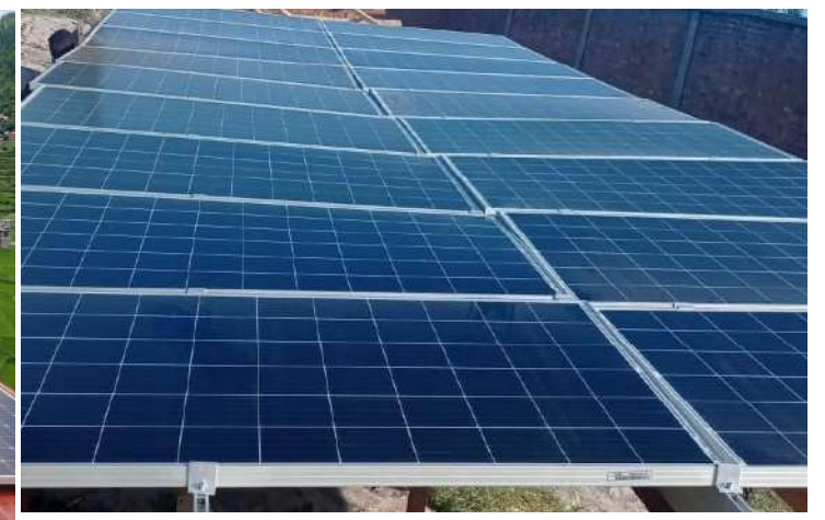
80 KW Solar Roofop Plant, Madagascar
