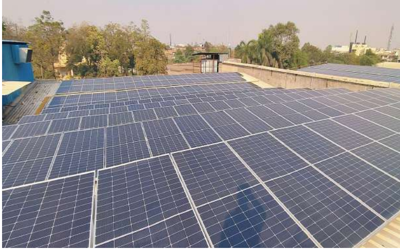
550 KW Solar Power Plant Ahmedabad, Gujarat
