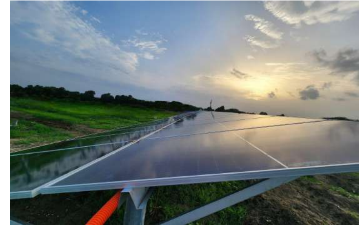
2.30 MW Solar Power Plant - Patan, Gujarat
