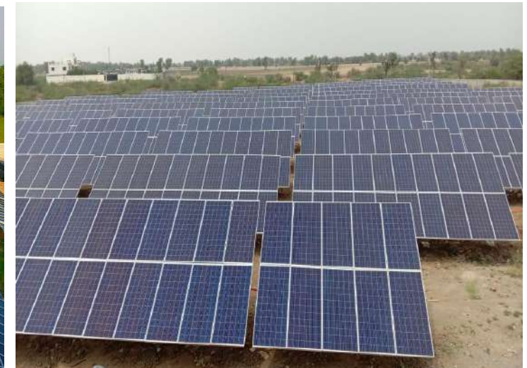
990 KW Solar Power Plant, Ahmedabad, Gujarat
