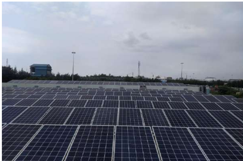
1 MW Solar Power Plant, Dahej, Gujarat
