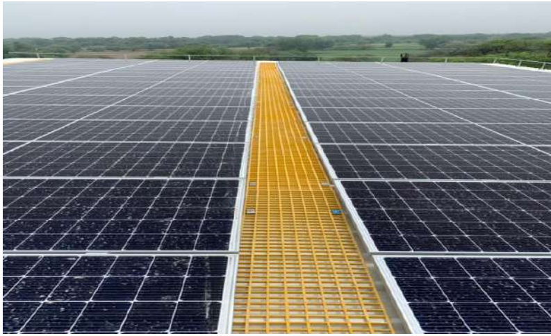
418 KW Solar Power Plant Kadi, Mehsana, Gujarat
