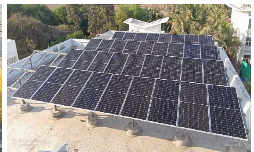
600 KW Solar Power Plant, Vavol Gandhinagar, Gujarat
