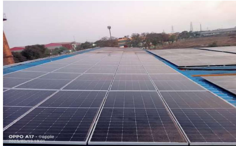
395 KW Solar Power Plant Narol, Gujarat
