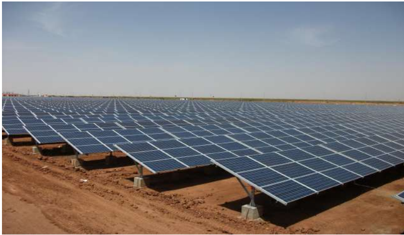
15 MW Solar Power Plant Surendranagar, Gujarat
