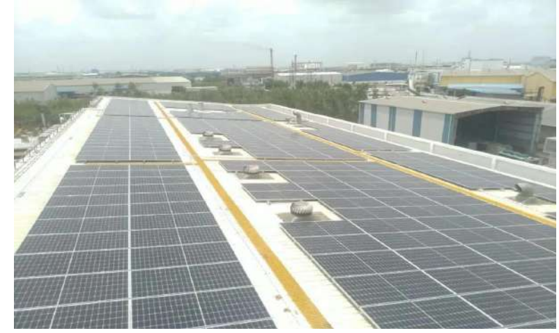
437 Solar Power Plant Sanad, Ahmedabad, Gujarat
