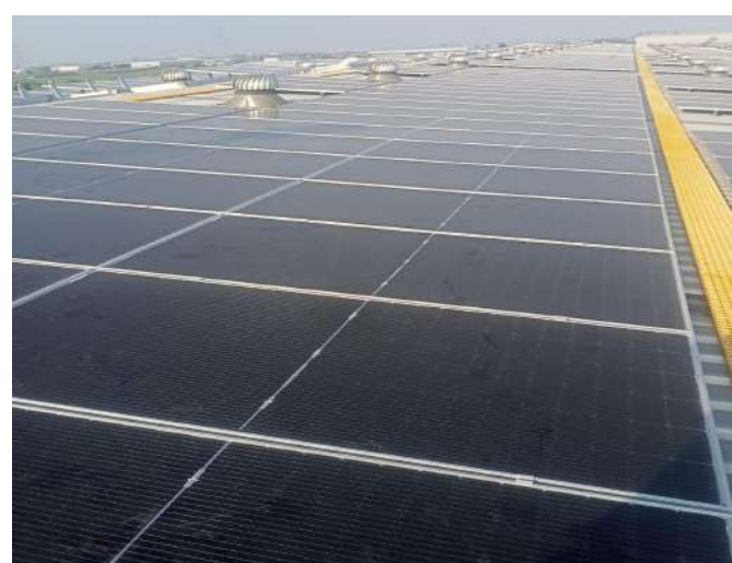
1.25 MW Solar Power Plant, Kheda, Gujarat
