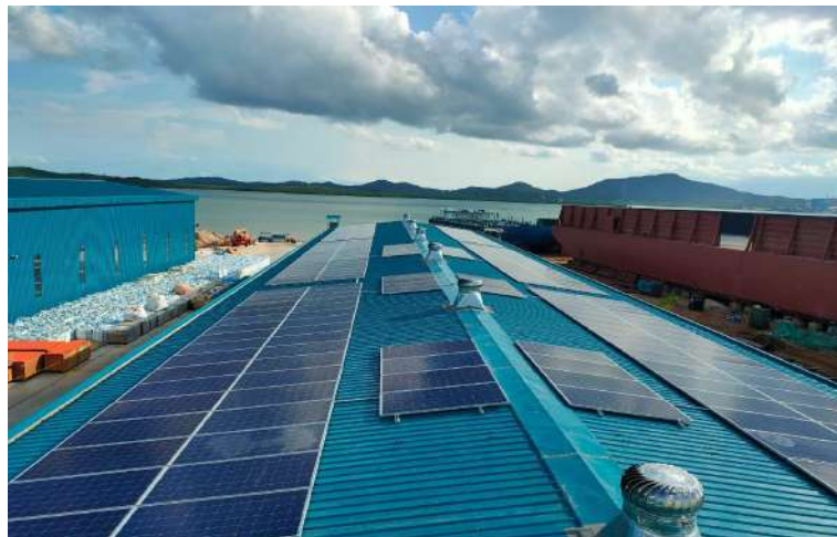
100 KW Solar Power Plant Indonesia
