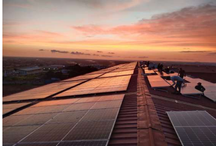
2.1 MW Solar Rooftop Power Plant West Africa
