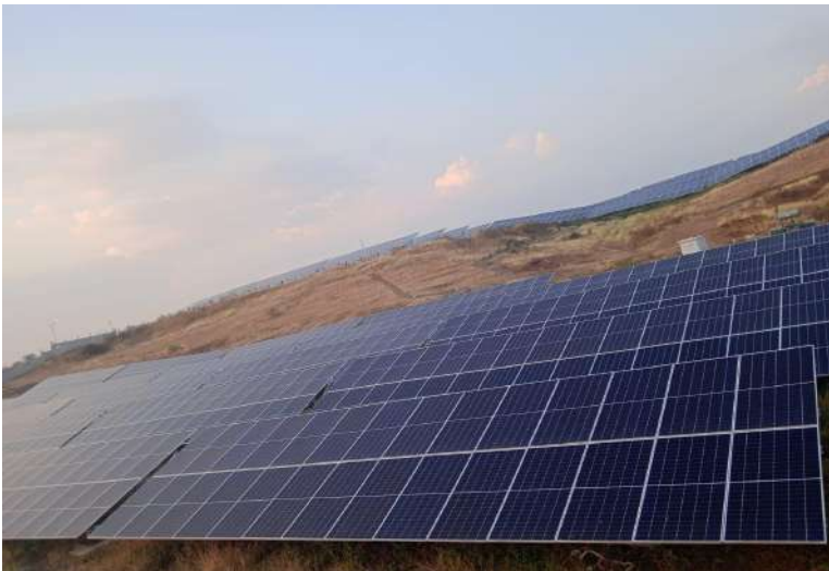
3.30 MW Solar Power Plant, Nasik, MH
