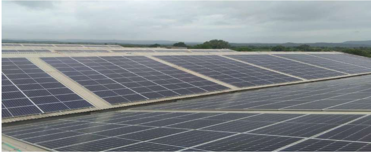
1 MW Solar Power Plant Burhanpur, Madhya Pradesh
