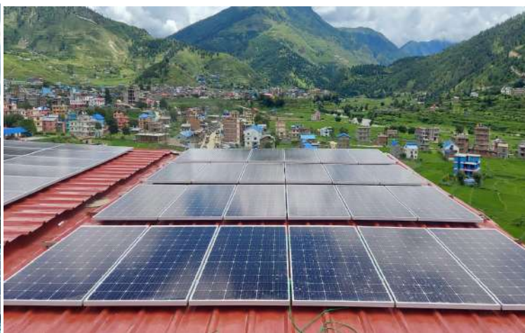
40 KW Solar Roofop Plant, Nepal
