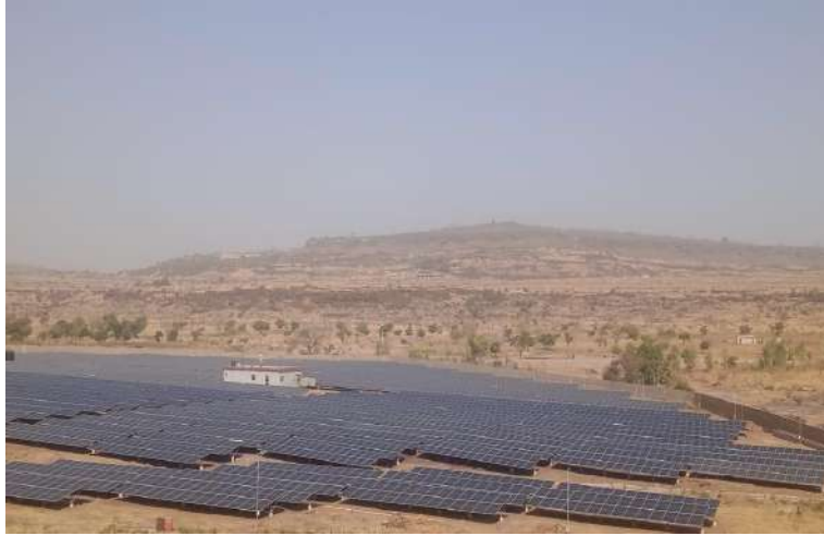
4.2 MW Solar Rooftop Power Plant Mali, Africa
