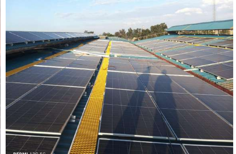
2 MW Solar Rooftop Power Plant Africa
