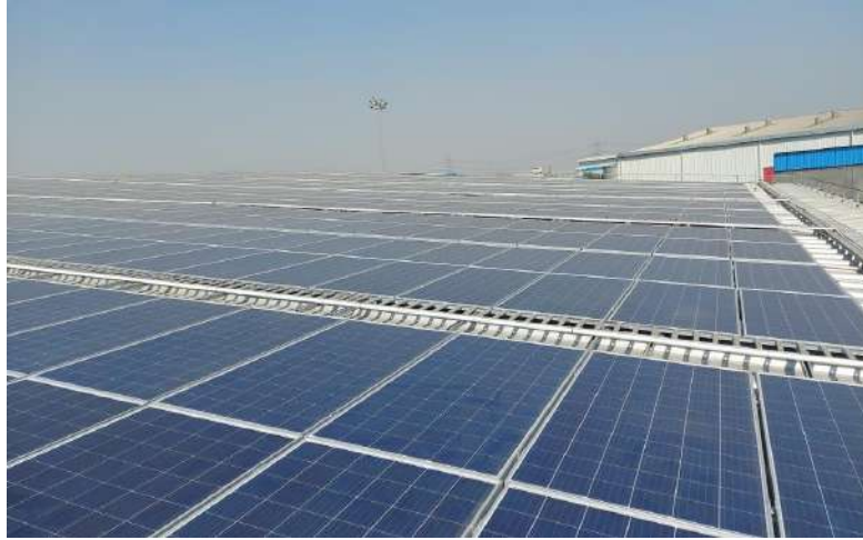
4 MW Solar Power Plant Bareja, Gujarat
