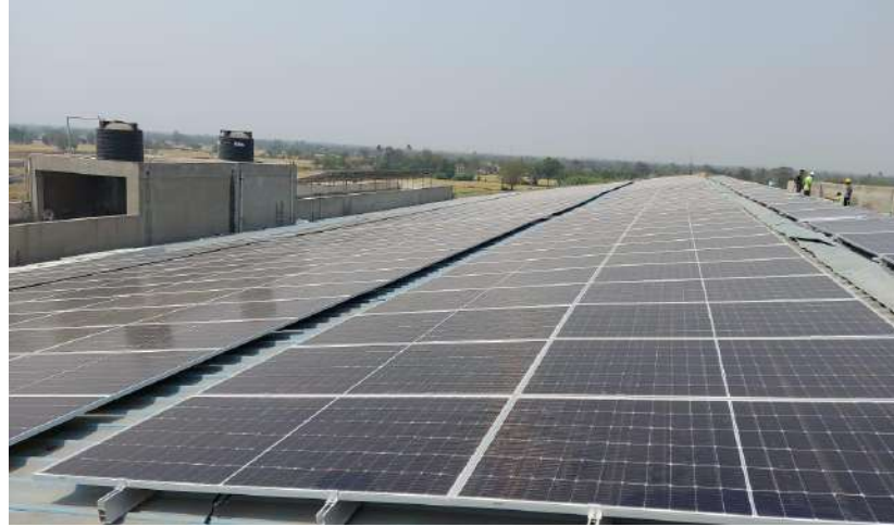
530 KW Solar Power Plant Paldi, Kankaj, Gujarat
