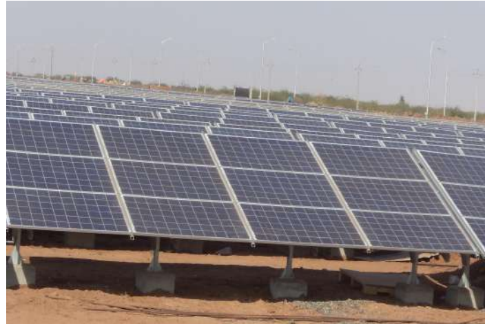
5.0 MW Solar Power Plant - Santalpur, Gujarat
