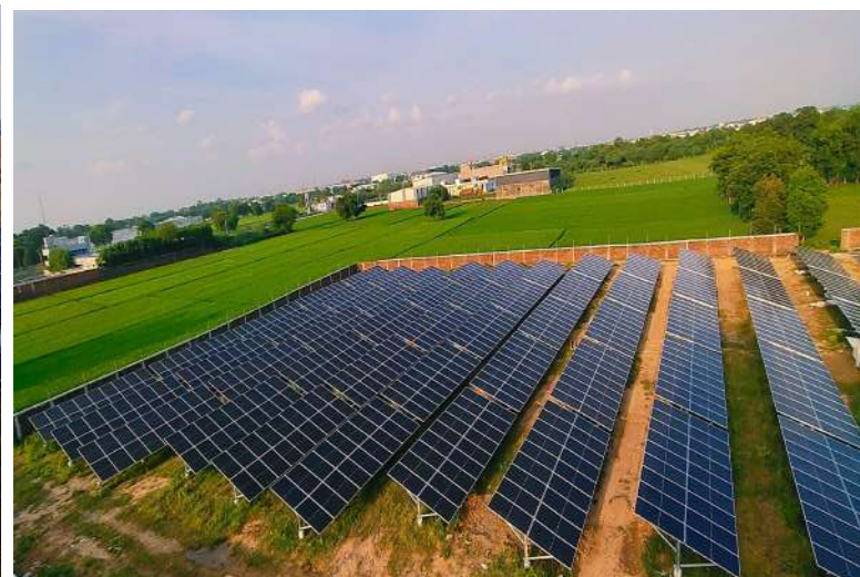
1.35 MW Solar Power Plant, Paldi-Kankaj, GJ
