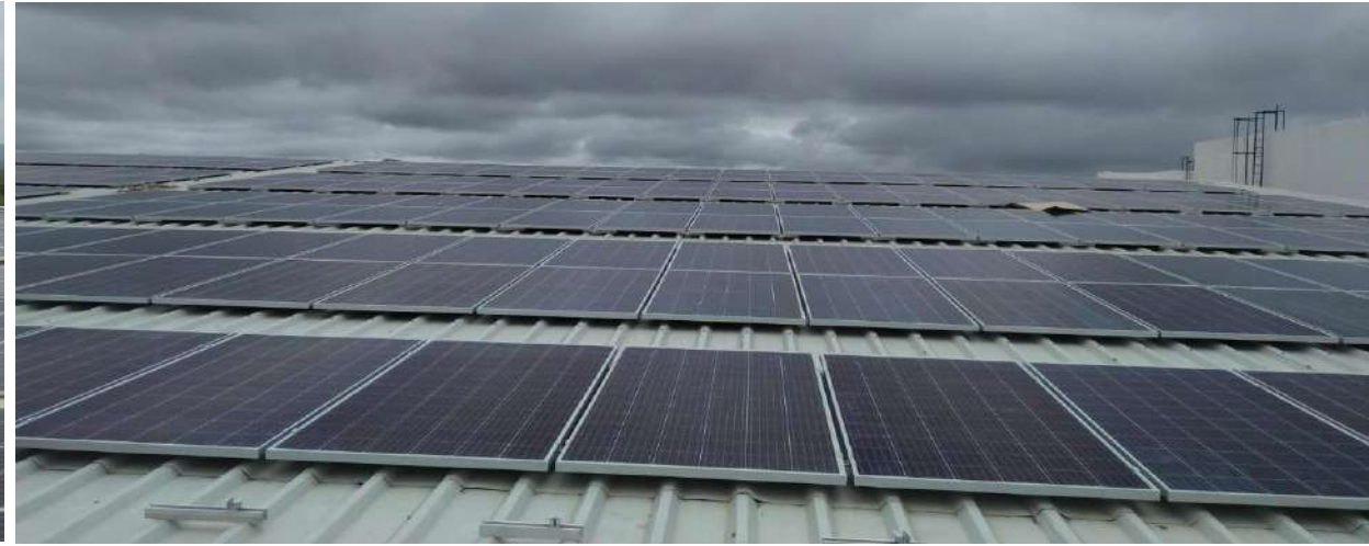
510 KW Solar Power Plant Nashik, Maharashtra
