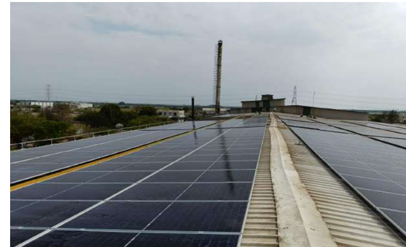
300 KW Solar Power Plant Kheda, Gujarat
