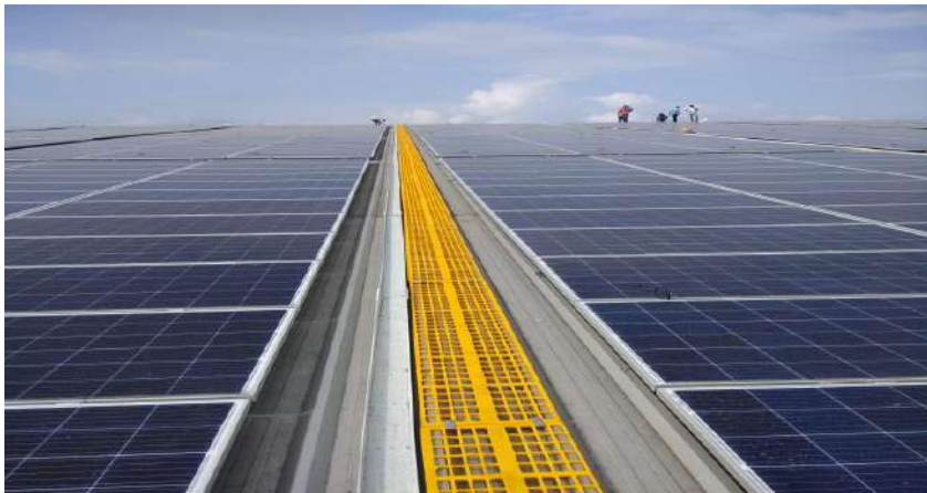
1200 KW Solar Power Plant Indore, Madhya Pradesh
