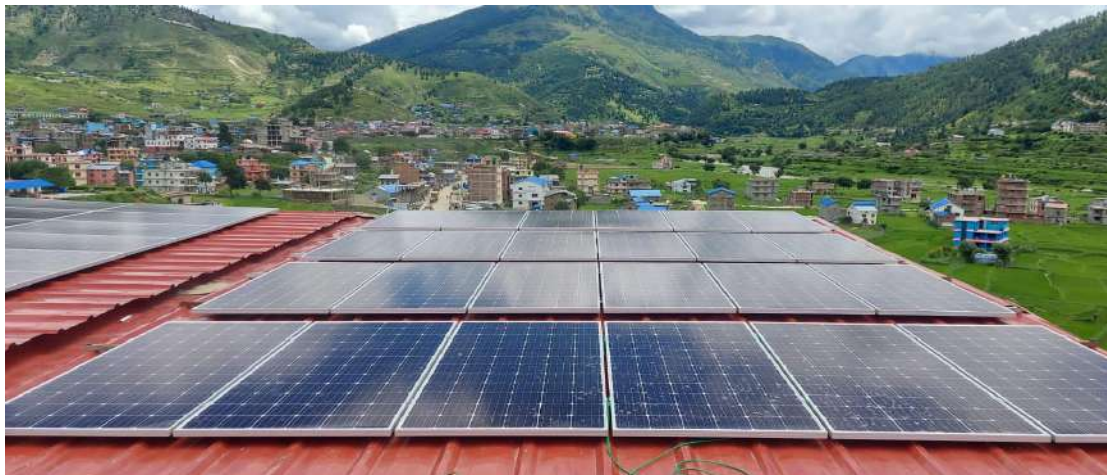
40 KW Solar Roofop Plant, Nepal
