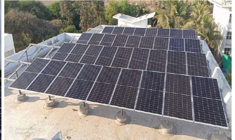
600 KW Solar Power Plant Vavol Gandhinagar
