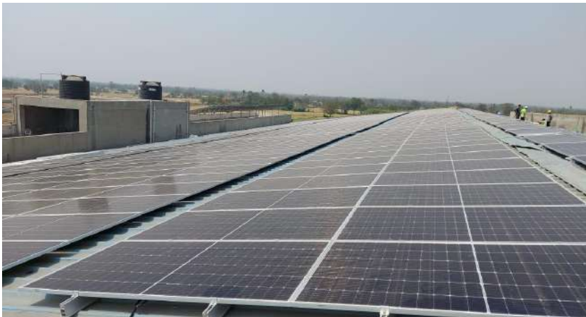
530 KW Solar Power Plant Paldi, Kankaj
