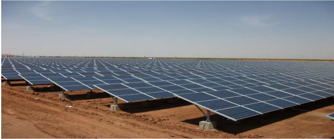
15 MW Solar Power Plant Surendranagar
