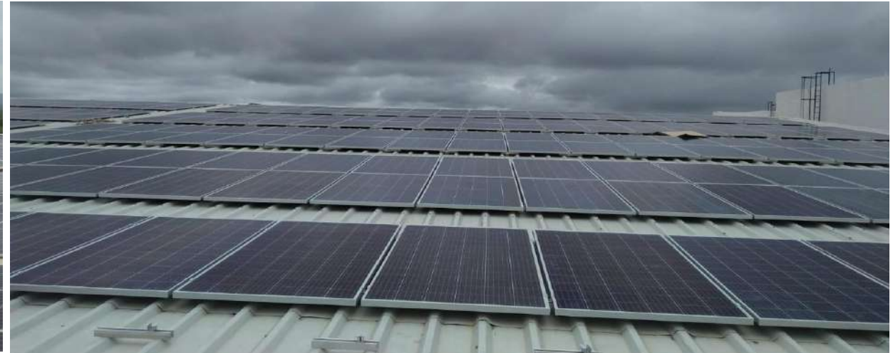
510 KW Solar Power Plant Nashik, Maharashtra
