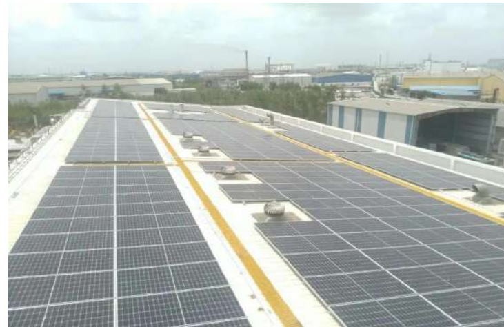
437 Solar Power Plant Sanad, Ahmedabad
