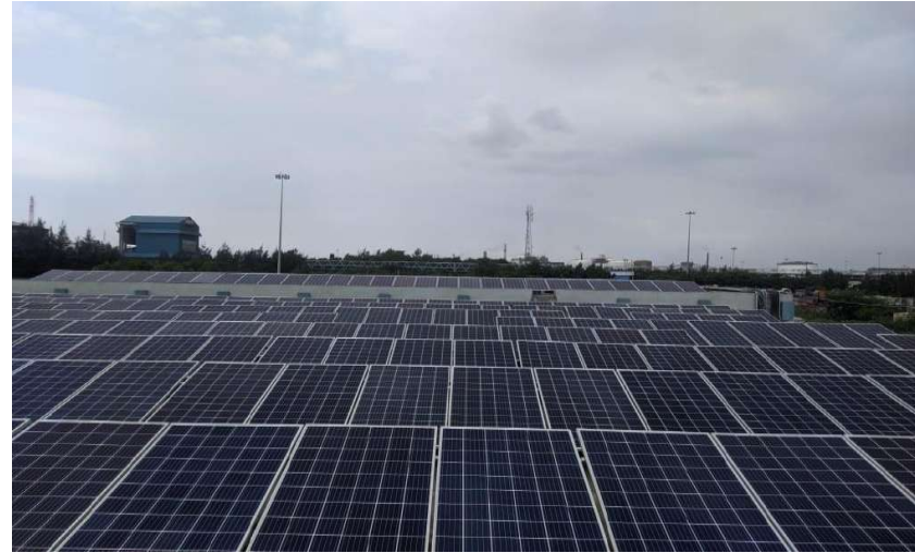
1 MW Solar Power Plant Dahej, Gujarat
