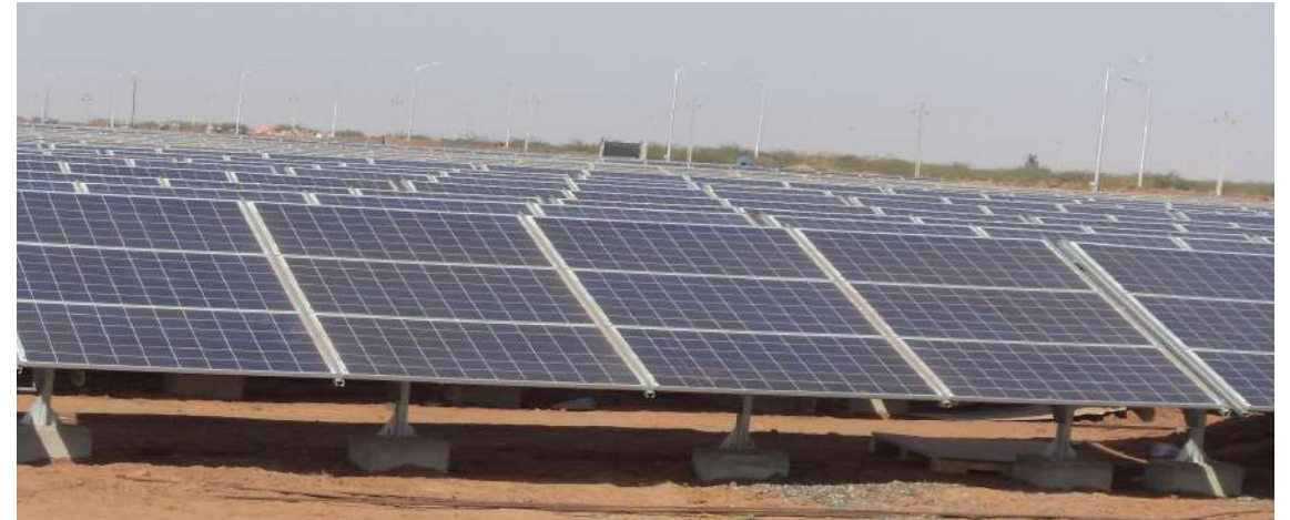
5 MW Solar Power Plant - Santalpur
