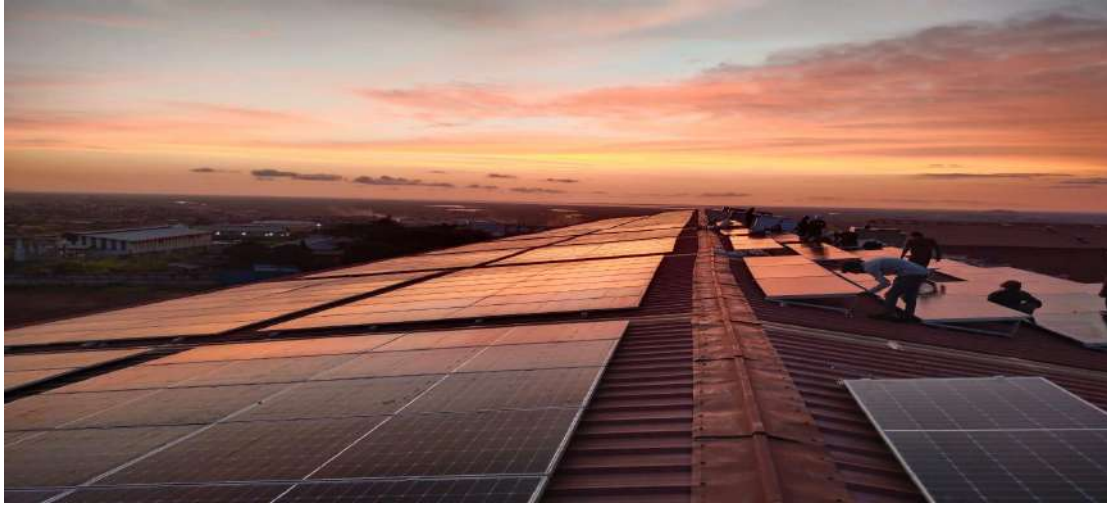
2.1 MW Solar Rooftop Power Plant West Africa
