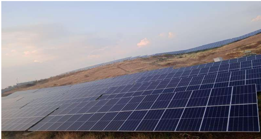
3.3 MW Solar Power Plant, Nasik, MH
