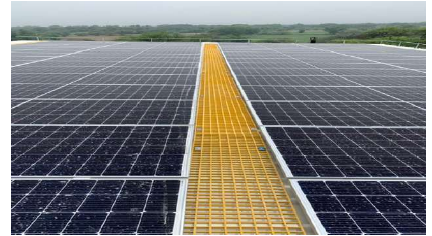
418 KW Solar Power Plant Kadi, Mehsana
