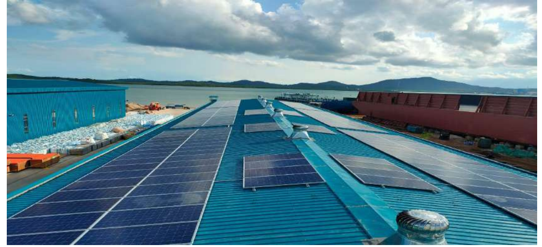
100 KW Solar Power Plant FMSI Service Inc.- Indonesia
