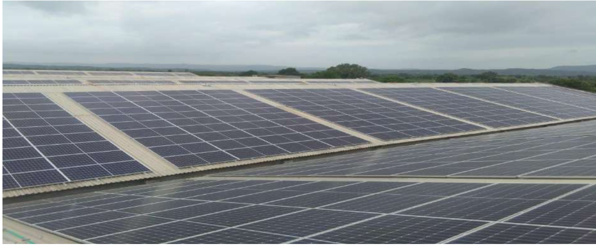
1 MW Solar Power Plant Burhanpur, Madhya Pradesh
