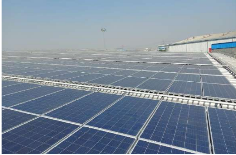
4 MW Solar Power Plant Bareja, Gujarat
