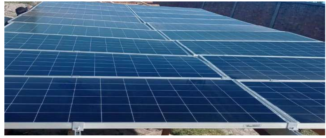
80 KW Solar Roofop Plant, Madagascar
