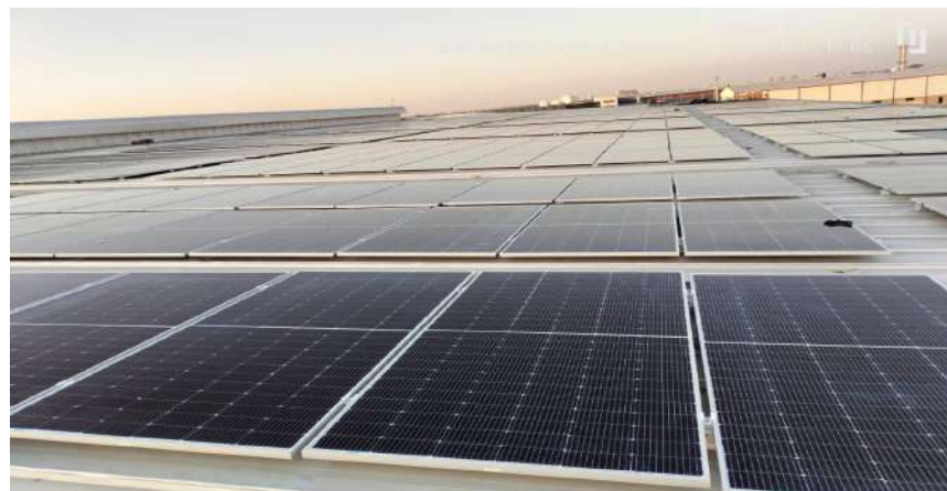
600 KW Jaipur, Rajasthan
